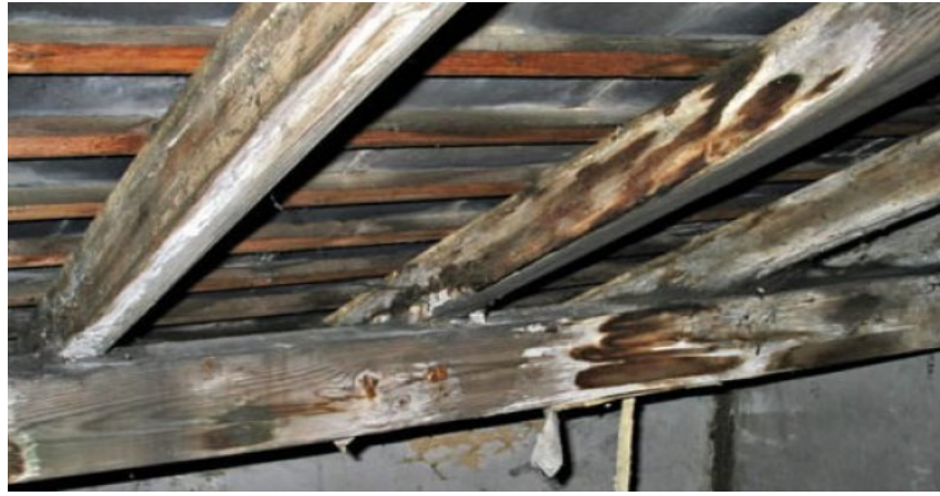
1. Roof Supporting Members with Water Damage.
