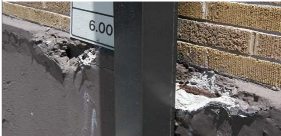
3. Typical Distress: Crumbling Foundation Wall and Exposed Rebar
