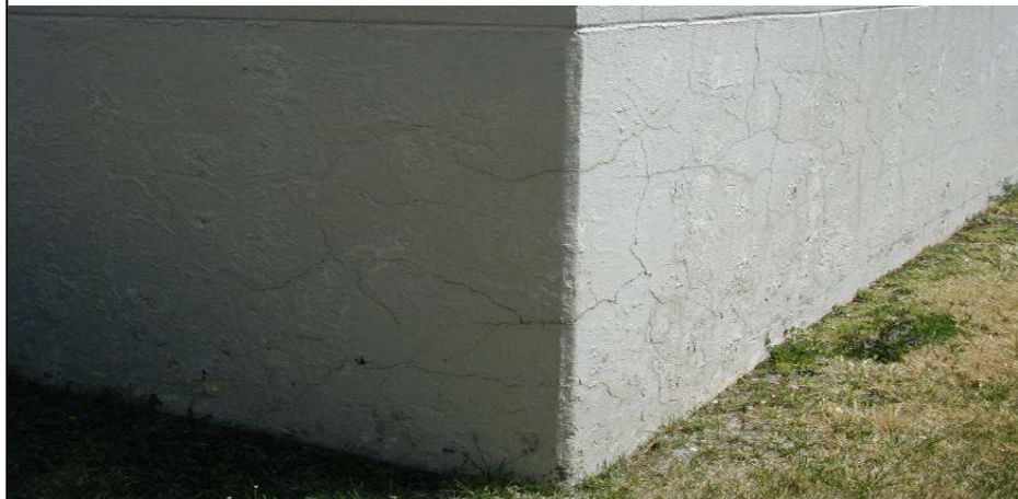
5. Typical Distress: Foundation Cracks
