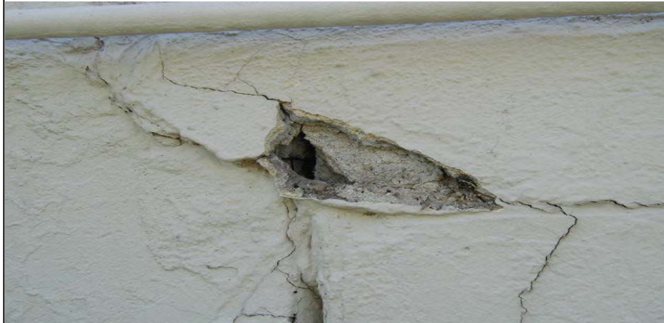
4. Typical Distress: Foundation Cracks & Spalls
