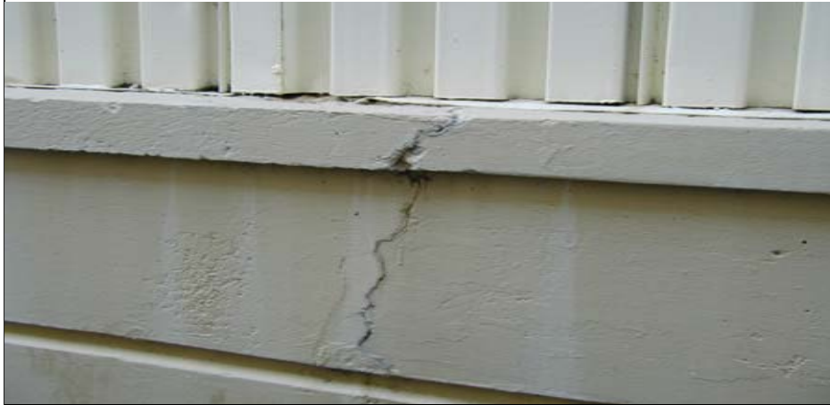
1. Typical Distress: Cracked Foundation Wall
