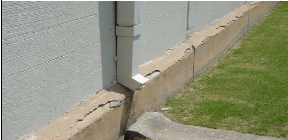
6. Typical Distress: Spalling Concrete Foundation
