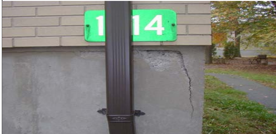
2. Typical Distress: Cracked Foundation
